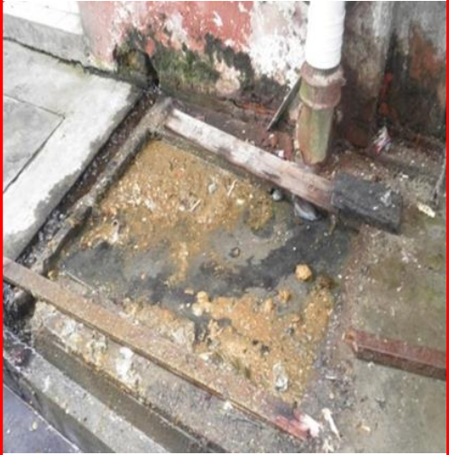
Untreated septic sludge
